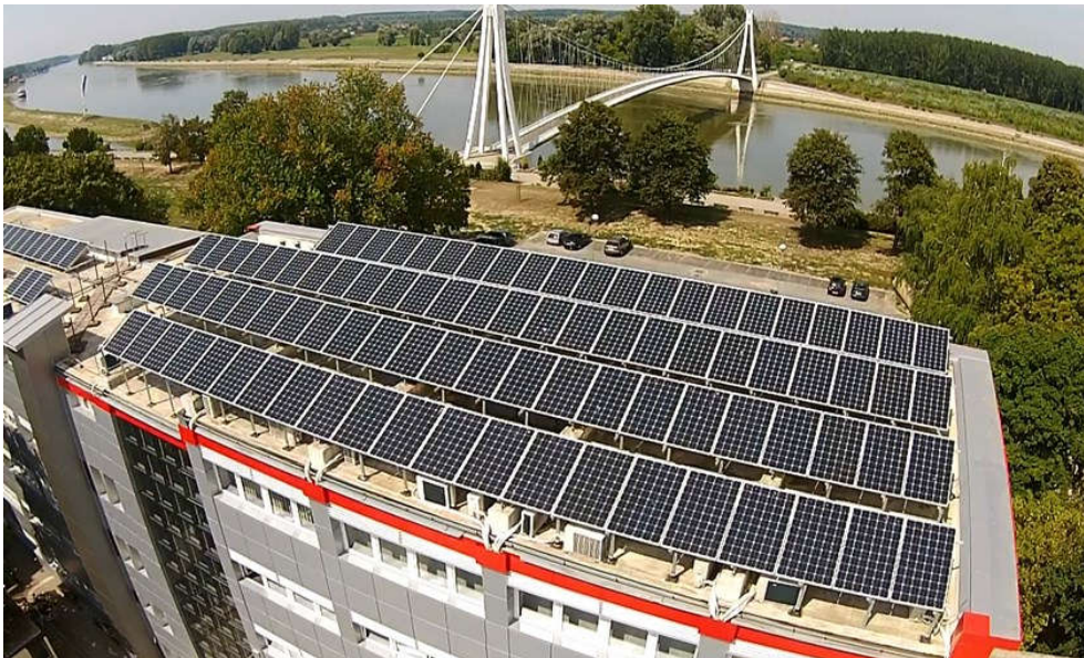
Figure 2-6 Example of integrated photovoltaic 29.64 kW power plant realization (source: HEP)
