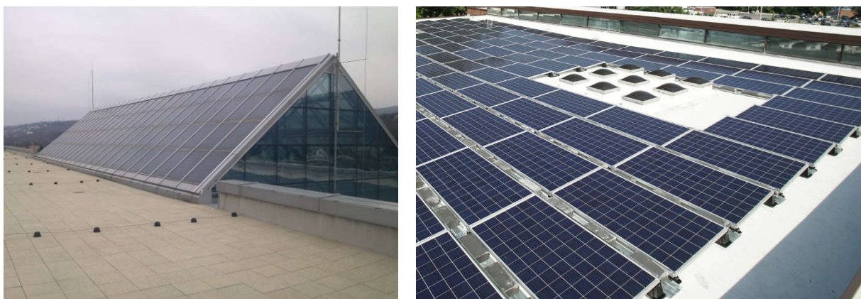
Figure 1-2 An example of a PV system integrated into a building and a PV system on flat roof
